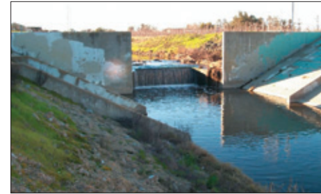
Figure 13 – The Marsh Creek Grade Control Dam Upstream of the Brentwood Wastewater Treatment Plant
