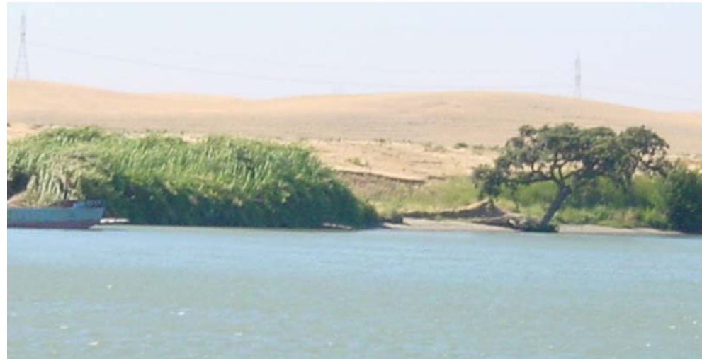
An established breach on the exterior of a breached levee
