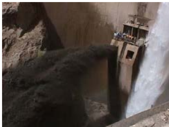
Figure 8: A flushing flow being released from a bottom outlet in Jiroft, Iran. Source: Schleiss 2008
